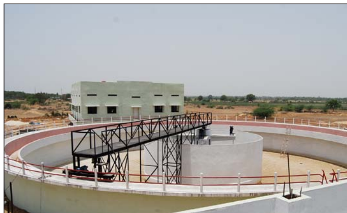
Clarifloculator at Gajwel Phase-I Project.
