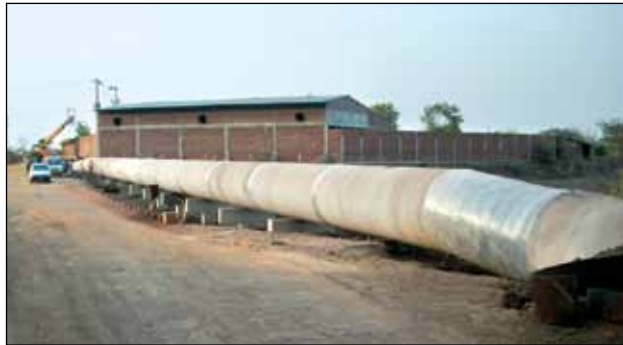
1700 mm dia x 10 mm thick M.S. Pipe Line with shrink wrap for curing for Raipur Augmentation WSS in Chattisgarh State
