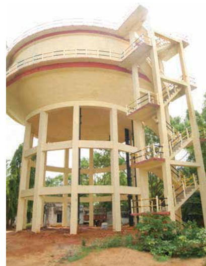
Elevated Storage Reservoir of 8 Lakh Liter Capacity
