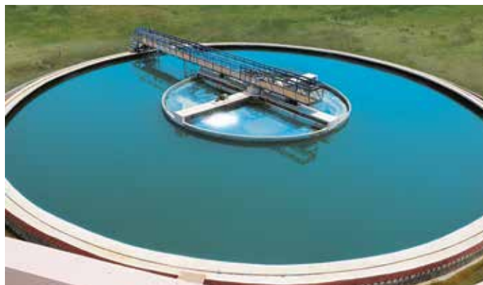
Clariflocculator at Dharmavaram Water Supply Scheme
