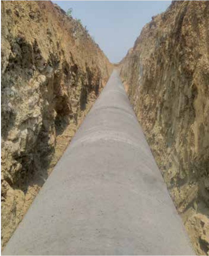
1000 mm dia PCCP Pipeline laying at Dighori Branch for Asolamendha Project, in Maharashtra
