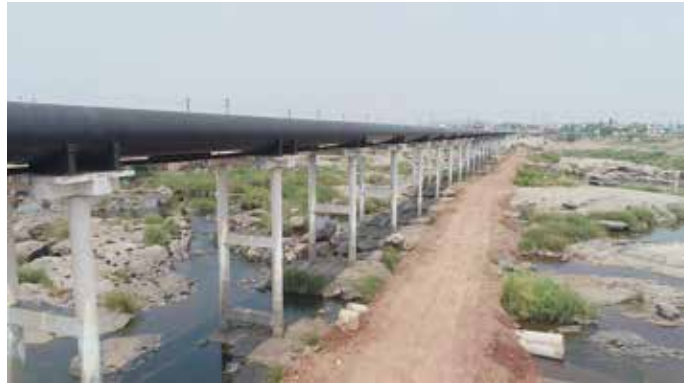
1600 mm dia MS pipeline laying for KPCL Bellary project for a length of 700 mtrs on existing bridge for crossing Tungbhadra River at Hospet, in Karnataka
