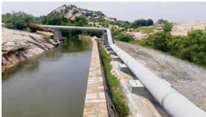
800 mm dia MS Pipeline for canal crossing for Alampalayam project, in Tamilnadu.
