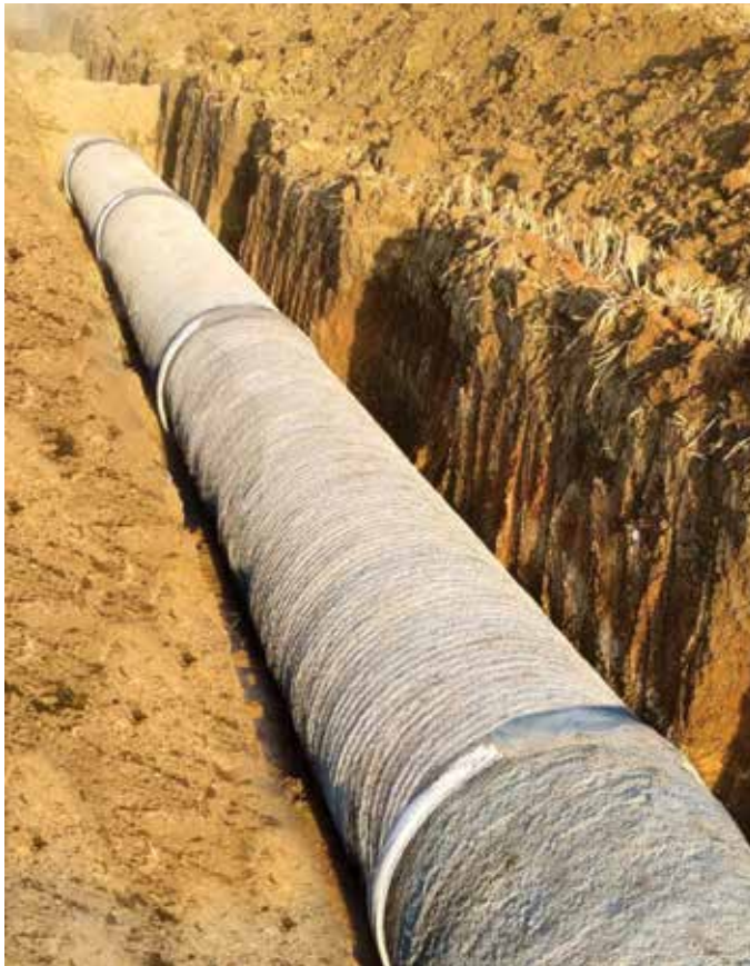
700 mm dia PCCP Pipeline laying at Pauni Lift Irrigation Scheme, in Maharashtra
