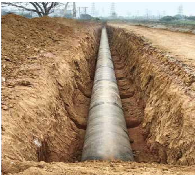
1500 mm Dia MS Pipeline laying work at Raw Water Gravity Main in Bilaspur Water Supply Scheme, in Chhattisgarh
